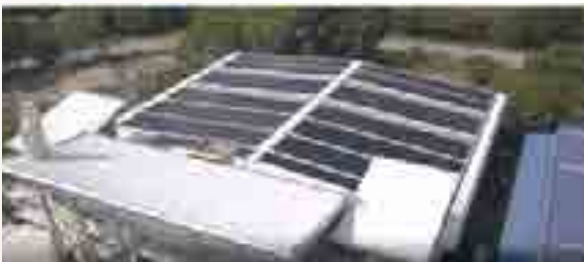
Figure 17: Solar Panel at NCT HQ Rooftop
